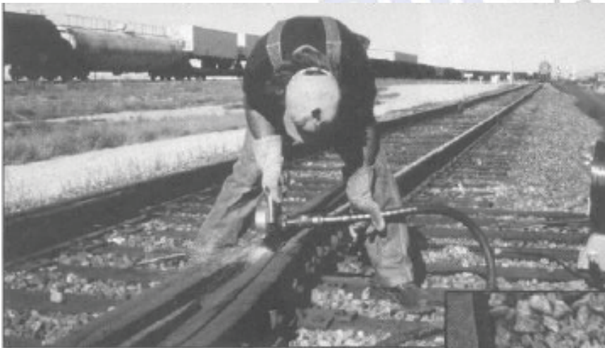
ABOVE: Finish grinding of a manganese steel frog after all welds have been completed.
