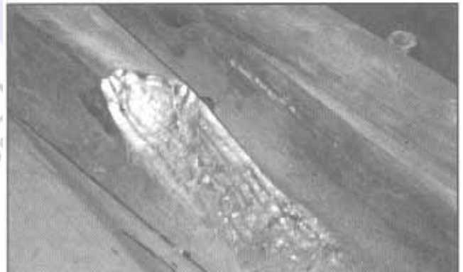
TOP: Air Arc Gouging of cracked frog point prior to welding. Welding equipment and air compressor mounted on welding truck.
