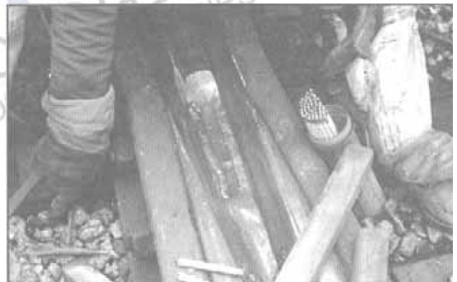
Build up of edges of flangeway point. To minimize heat buildup, narrow (stringer) beads are used. Note the Tempilsticks to check casting temperature.
