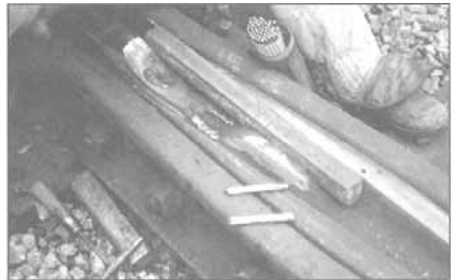
Rebuilding a frog point using Postalloy® FrogTuff-FCO wire. Use flangeway carbon (graphite) blocks inserted in flangeway opening to facilitate the build up of the point and wings. This practice is used to minimize the grinding of the flangeway side walls.
