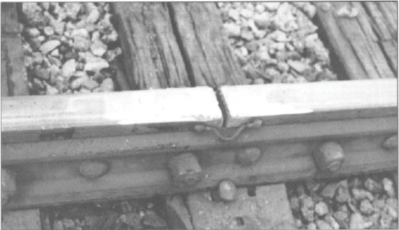
Correctly welded, ground, and cross slotted rail ends. Rail ends should be preheated to 700°F (367.4°C) and after welding post heated to 1100°F (587°C). Slow cool using cooling box to cover rail ends is recommended. Rail ends above were rebuild with Postalloy® RailTuff-FCO.
